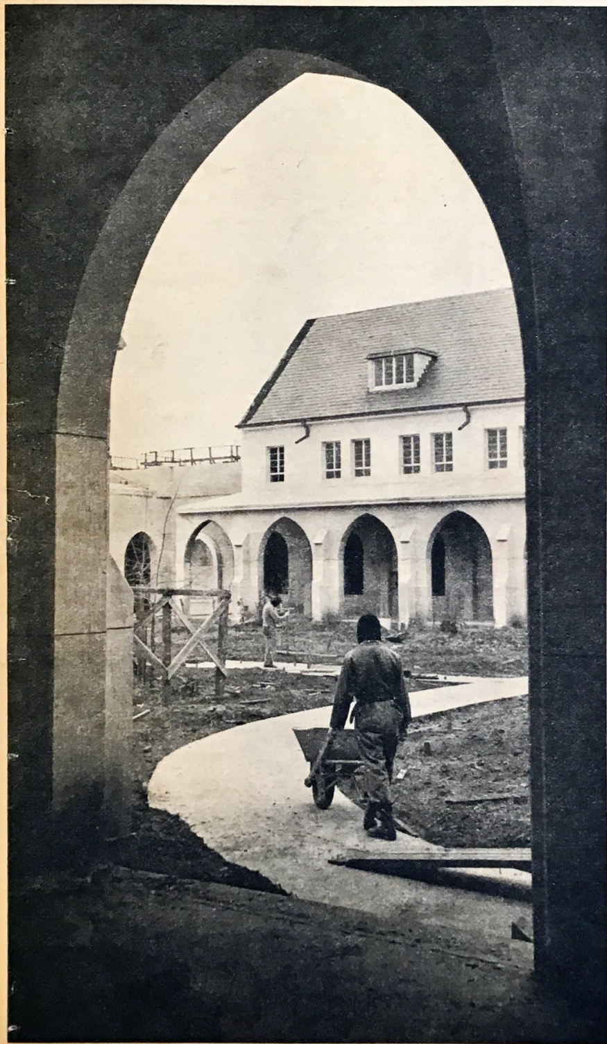
Here's a view of the cloister garden of the new Trappist monastery near Conyers, Ga.
