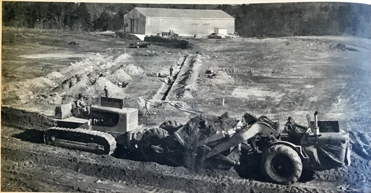
Red hills echo to the roar of work in progress at the site of Lockheed's multimillion-dollar A-plane research center near Dawsonville, Ga.
